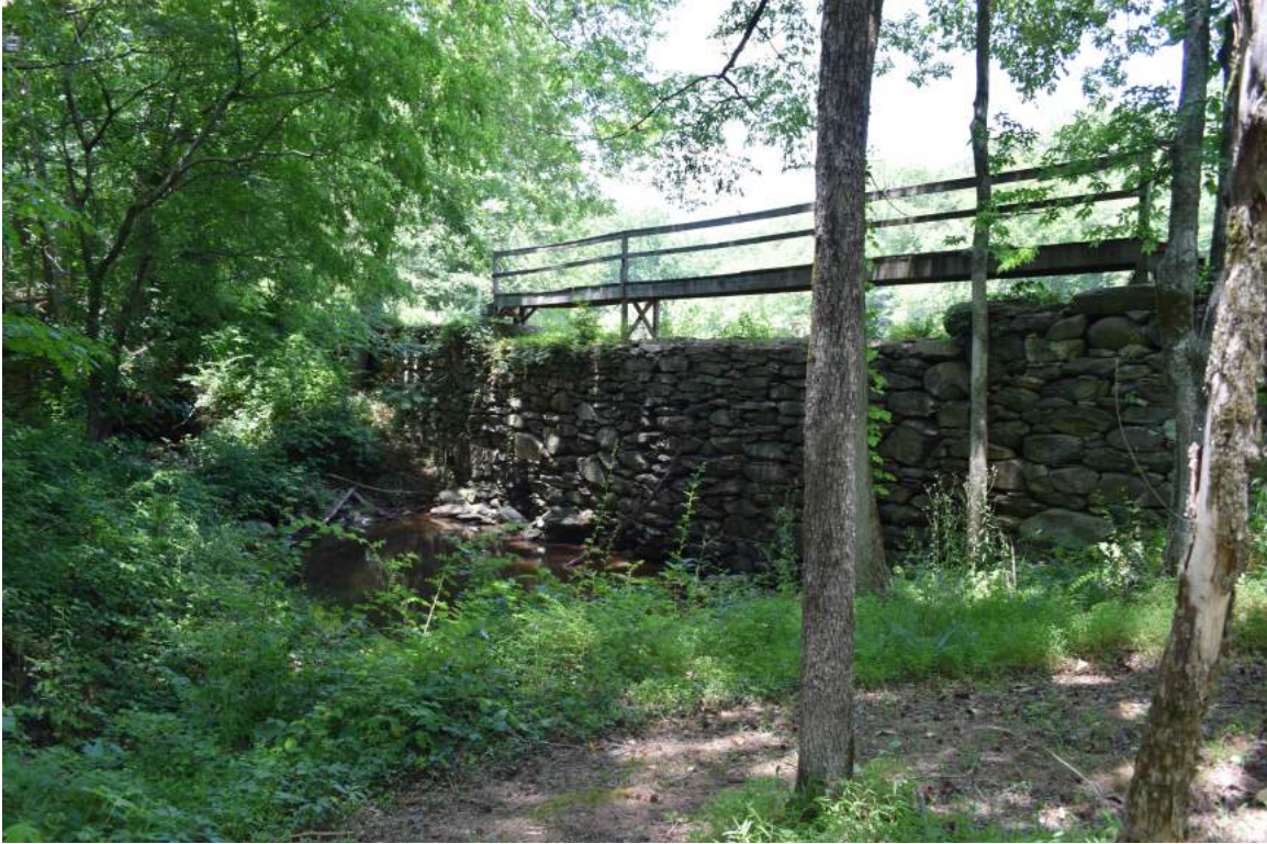
Faucett Mill Dam (OR0301), photographed by the authors June 2015 during the Orange County Architectural Survey Update.
