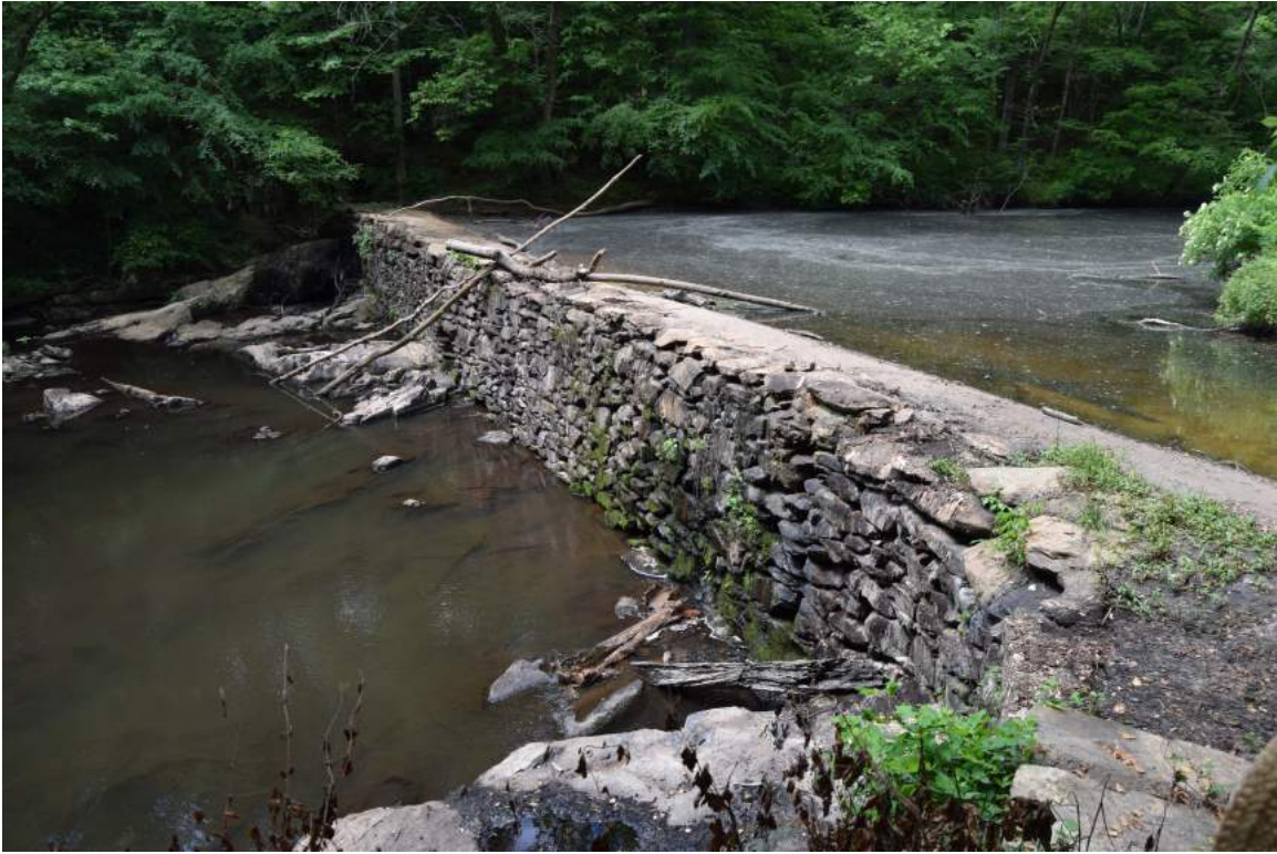
Morrow Mill Dam (OR0879), photographed by the authors June 2015 during the Orange County Architectural Survey Update.
